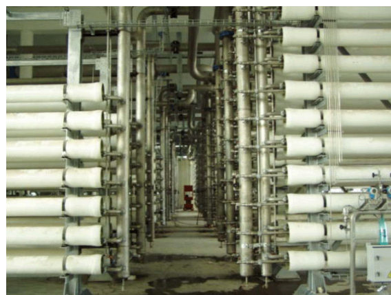
Fig. 7. Eupen RO plant under commissioning.
