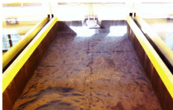
Fig. 5. Eupen sand filter washing.
