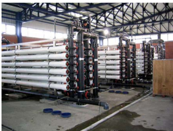
Fig. 7. UF units installed on site.
