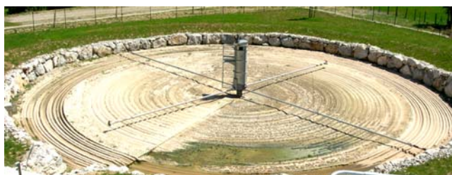
Fig. 6. Final sand filter with complementary safety volume in Roncal (Navarra).
