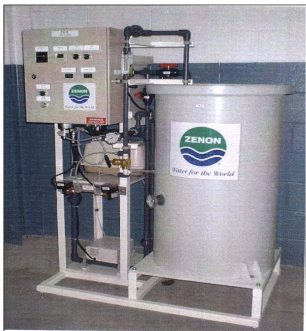
Fig. 1. Membrane bioreactor pilot module.
