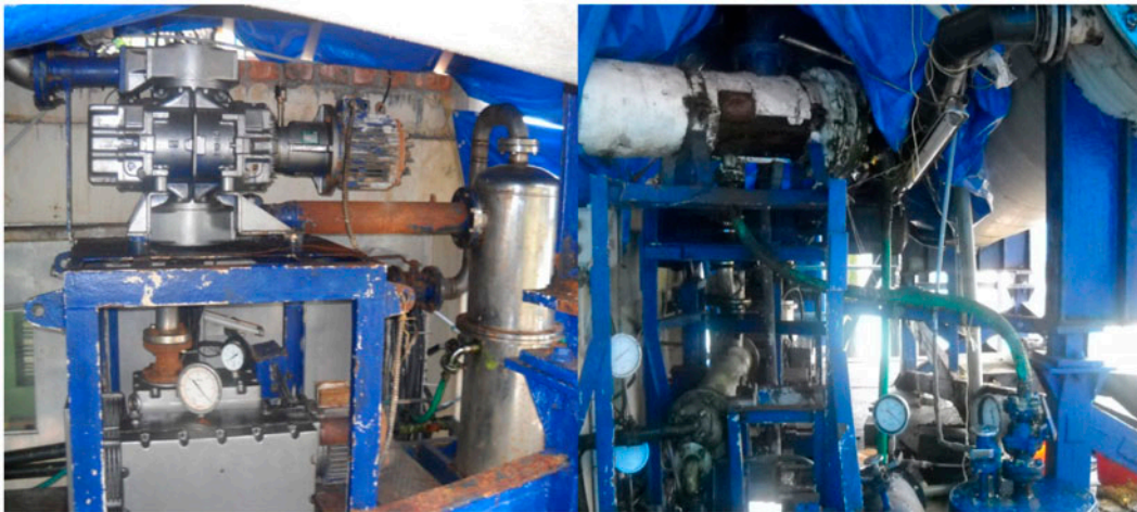
Fig. 15. Vacuum system in Kavaratti.
