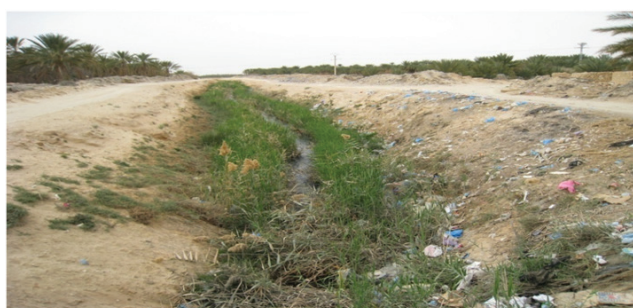
Fig. 14. Drainage ditches degraded due to lack of maintenance [10].
